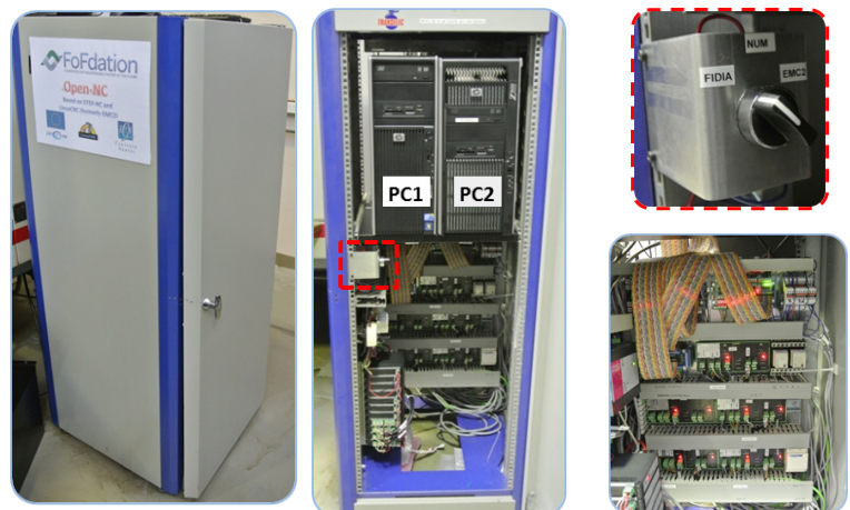
Figure 3: Prototype Platform - Electrical cabinet, LinuxCNC motion hardware, CNC source switch
